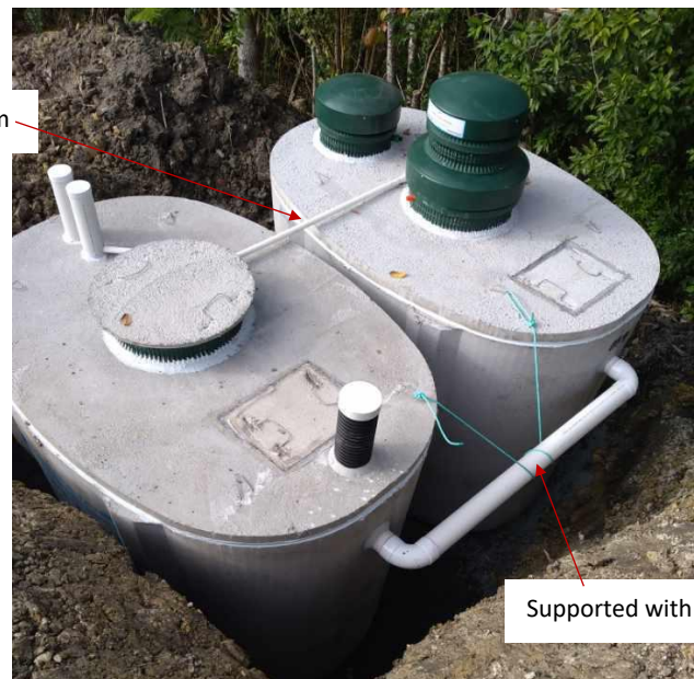
Sludge return 25mm
